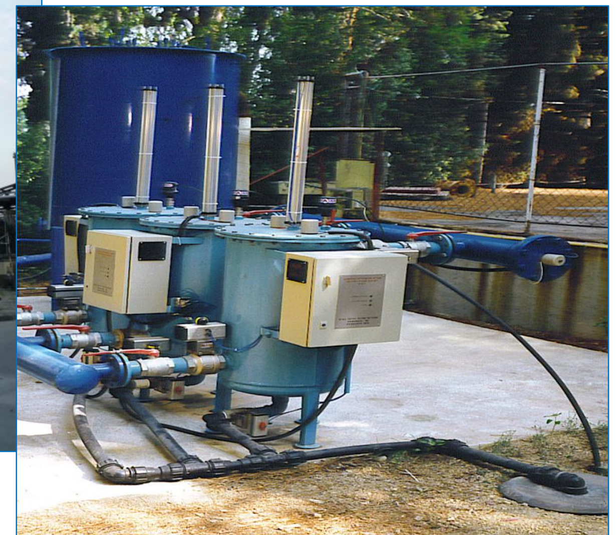
Disinfection of Well Water - Israel
