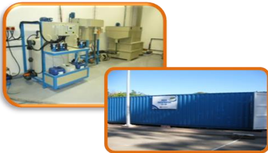
EEC system for heavy metal removal
