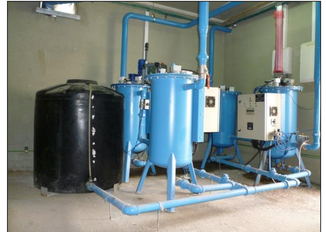
EST systems with a re-use water tank for irrigation
