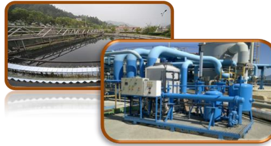
SWT- for the sewage cooling tower water treatment
