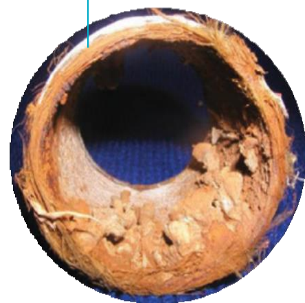
Corroded pipe with treatment
