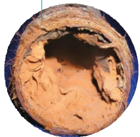
Corroded pipe without treatment
